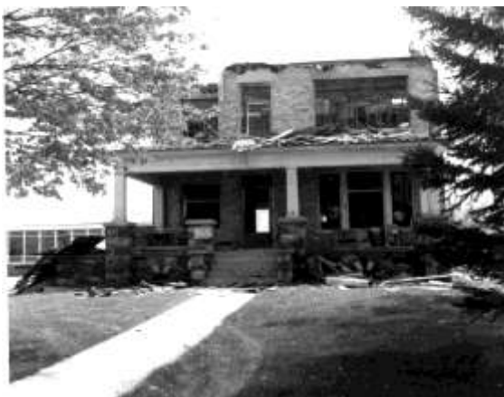
St Andrew old rectory demolished by men of the parish with the assistance of Louis Gruber, age 90, who helped build the rectory as an apprenticed
